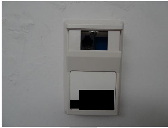
Typical BMS system sensor.
