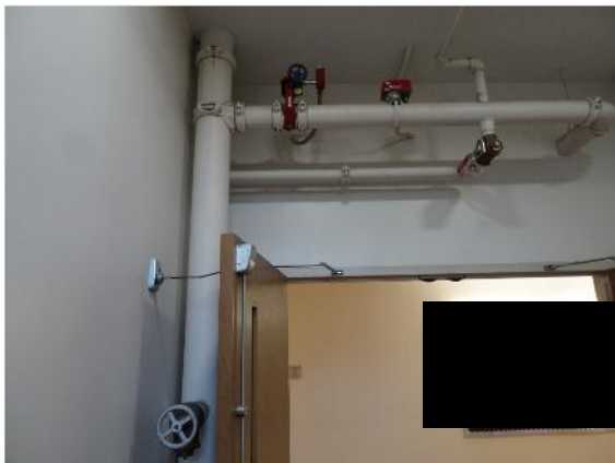
Typical stairway wet riser and sprinkler system control.
