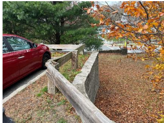
Leaning retaining wall adjacent parking lot along [REDACTED]
