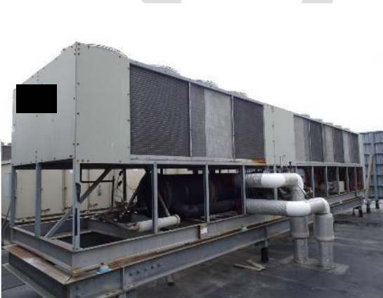
One of two roof mounted air cooled chillers.
