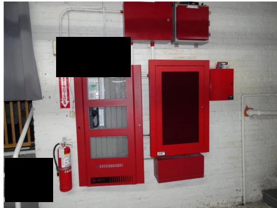
Main fire alarm panel.
