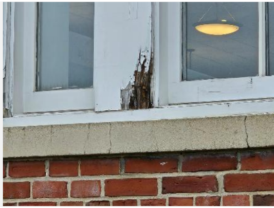
Deteriorated wood trim and cracked precast sill.
