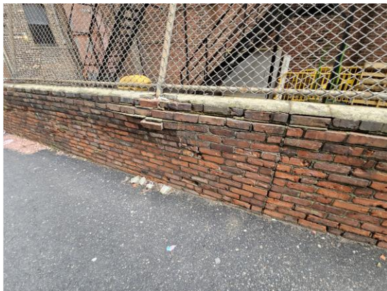
Alternate view of failed retaining wall.
