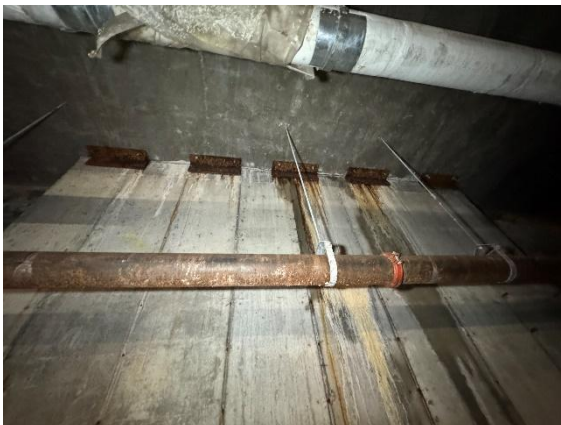
Water intrusion in sidewalk vault.
