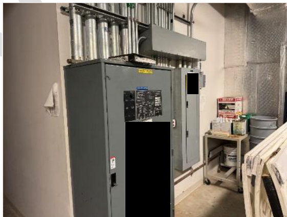
Automatic transfer switch.
