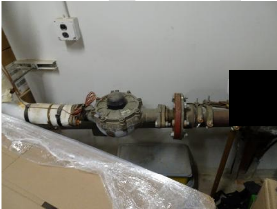
Domestic water main and meter.
