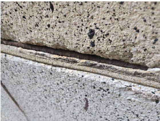
Spalled stone with exposed rebar.
