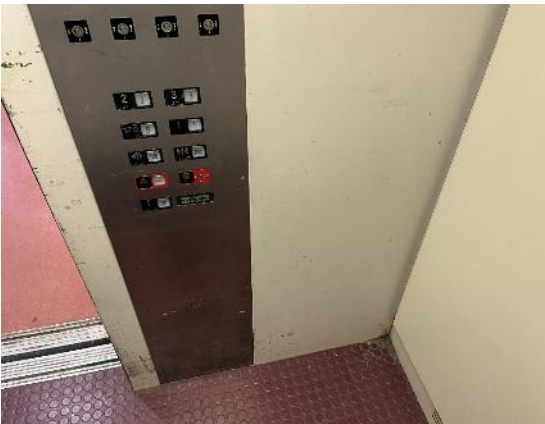
Elevator Car Station.
