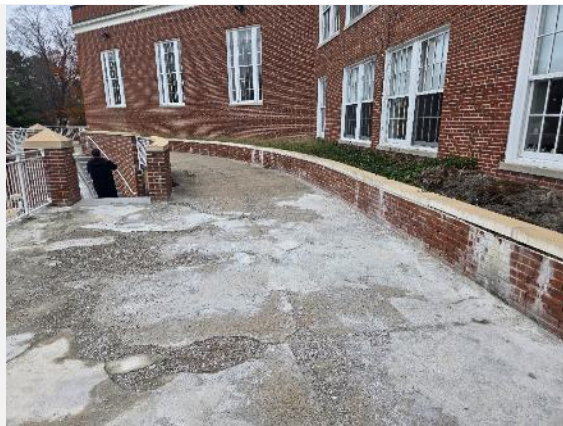
Damaged concrete deck over loading dock.
