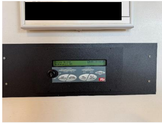
Fire alarm remote annunciator.
