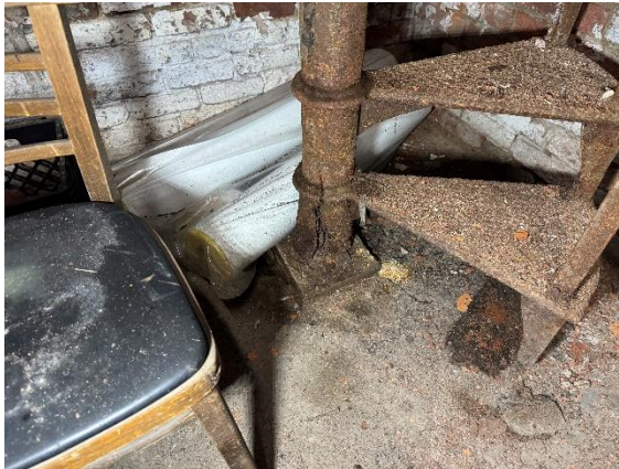
Deteriorated spiral staircase base.
