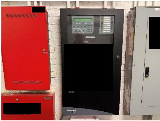
Fire alarm control panel.
