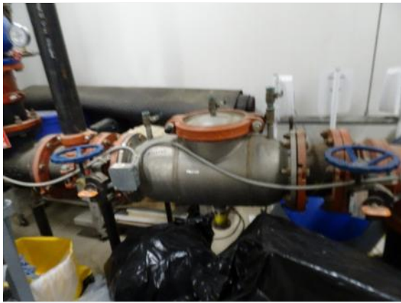
Fire protection main and backflow device.
