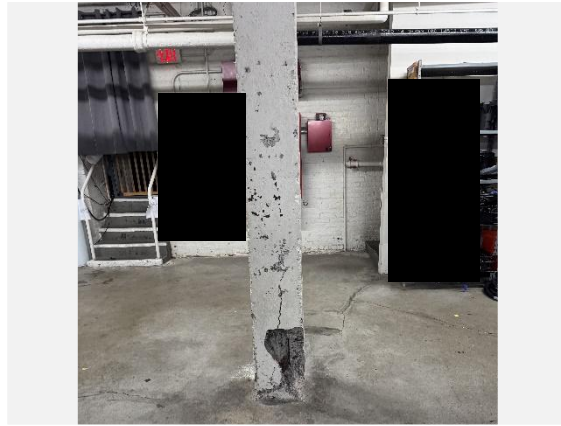
Typical rust jacking condition in basement columns.
