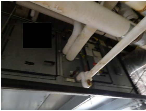
One of nine AHUs inside the building.
