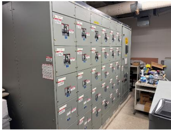
Electrical main switchboard.
