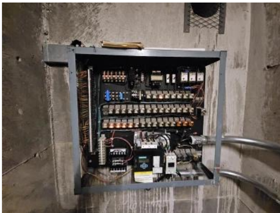
Freight Elevator Relay logic controller
