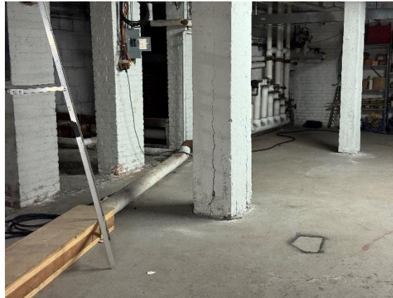
Typical rust jacking condition in basement columns.
