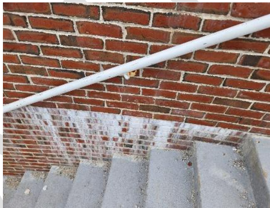
Efflorescence on brick.
