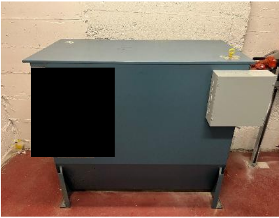
Elevator Power Unit.
