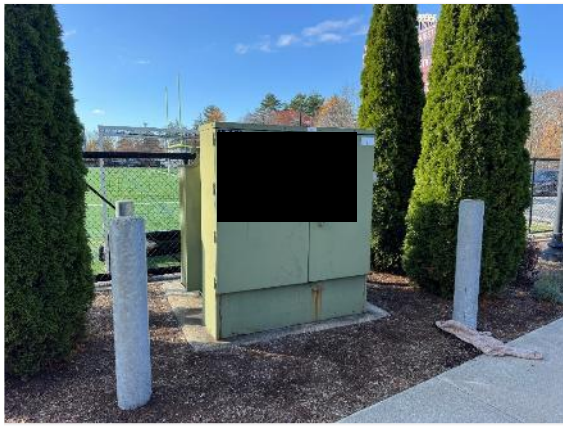
Electrical utility transformer.
