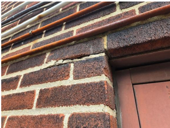
Failed mortar and rust jacking at lintels.
