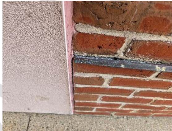
Crazing and failed sealant.
