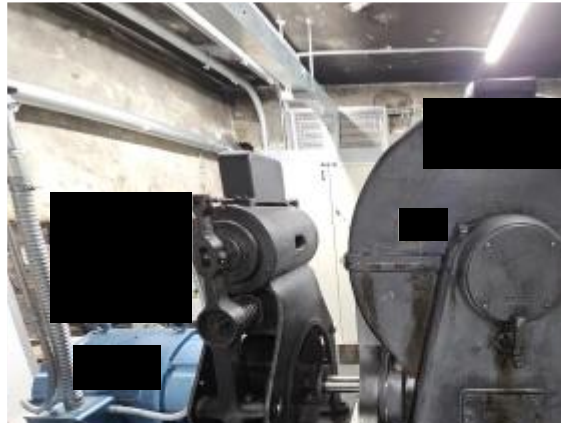
Passenger Elevator machine
