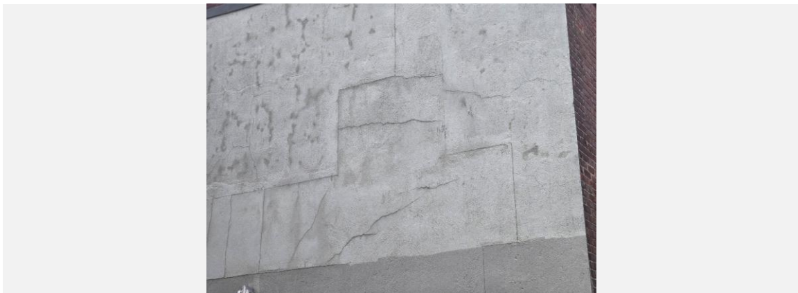
Cracked concrete parge coating.
