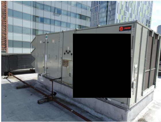
Typical HVAC rooftop unit.
