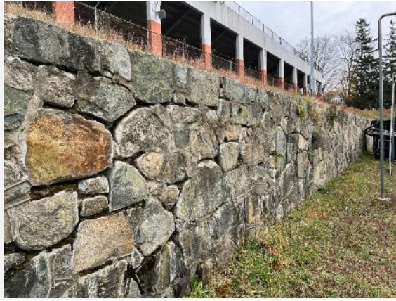
Degraded fieldstone wall between football and baseball fields.
