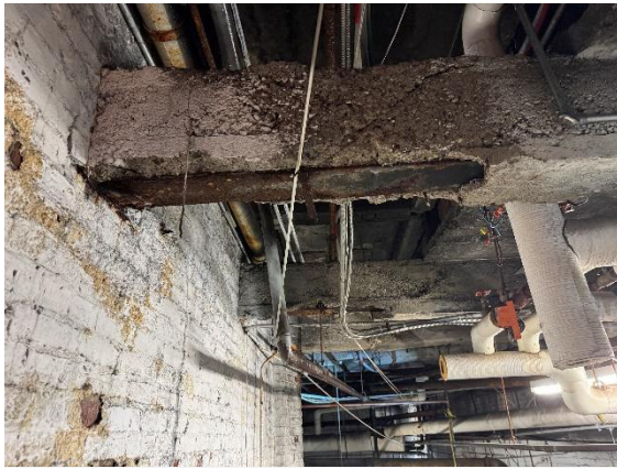
Typical beam deterioration in basement.
