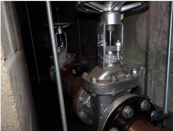
Domestic water main and meter.
