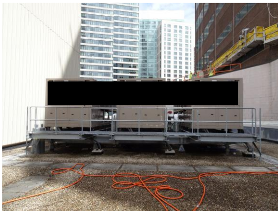
Air cooled chillers.
