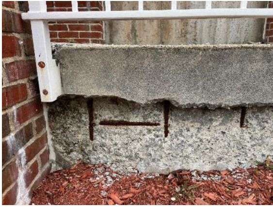
Degradation observed at main entryway concrete ramp.
