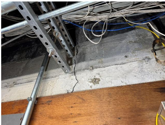
Settlement cracking in exterior foundation wall.
