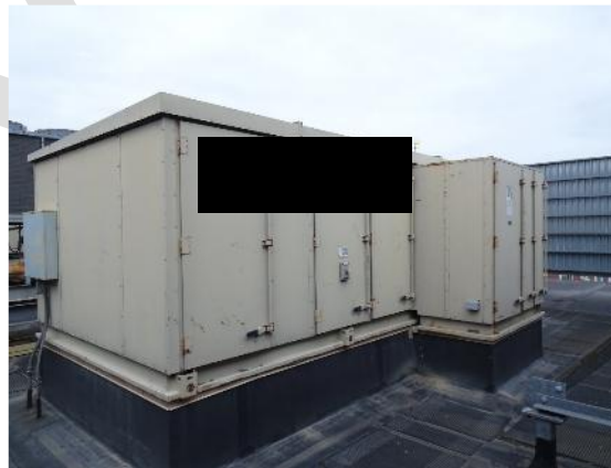
One of three roof mounted AHUs.
