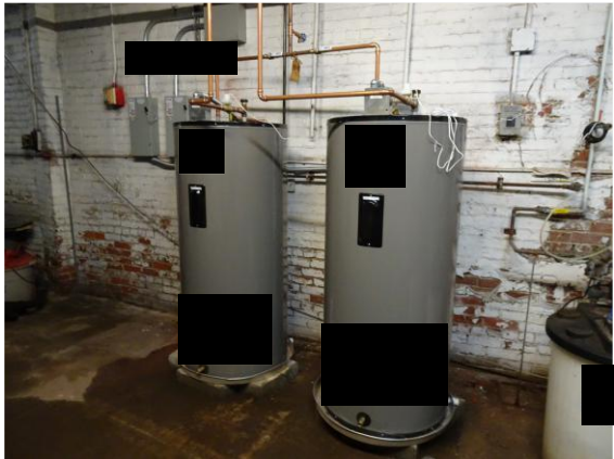
Domestic water heaters,
