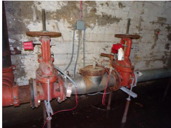
Fire protection main and backflow device.
