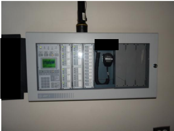
Fire alarm remote annunciator.
