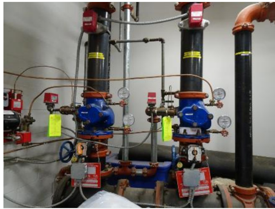
Sprinkler system risers.
