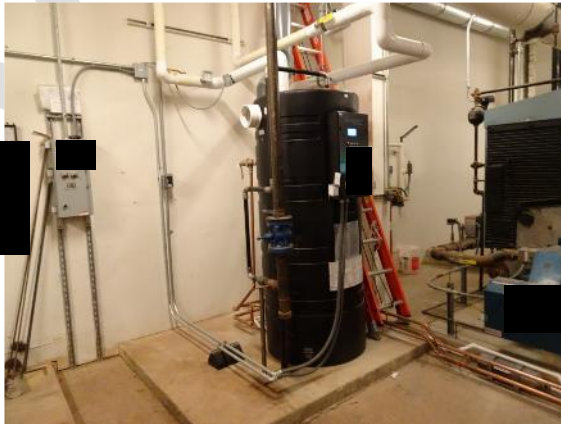
Main domestic water heater.
