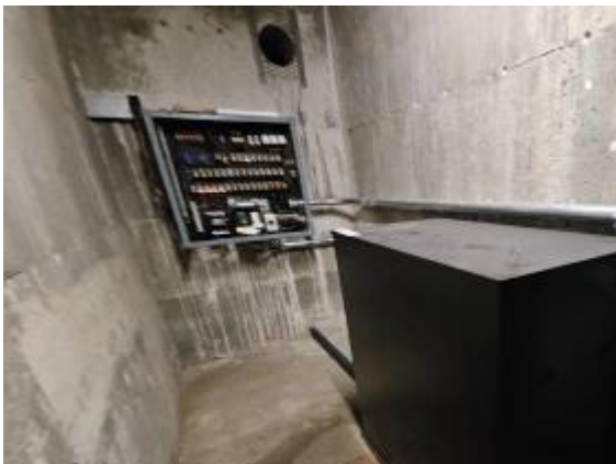
Freight Elevator Power unit
