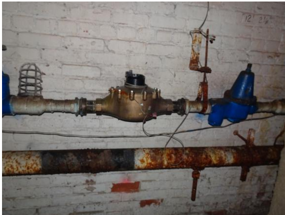
Domestic water main and meter.
