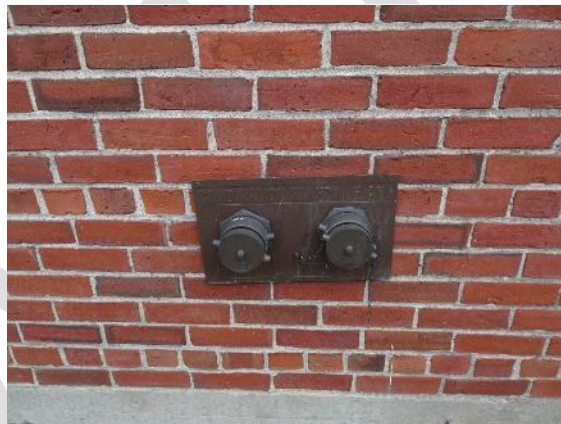
Exterior connection for fire department use.
