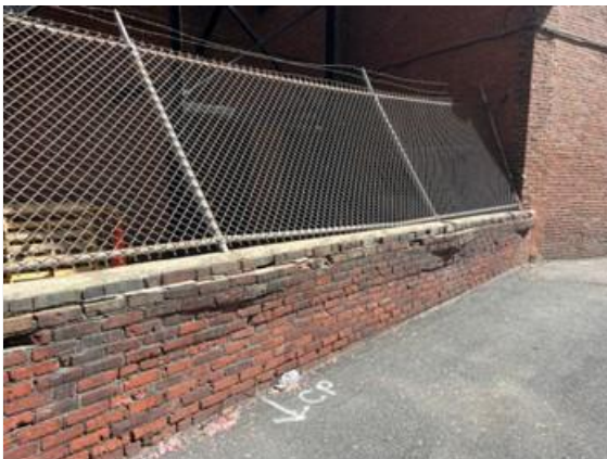
Bowing retaining wall and fencing along [REDACTED]
