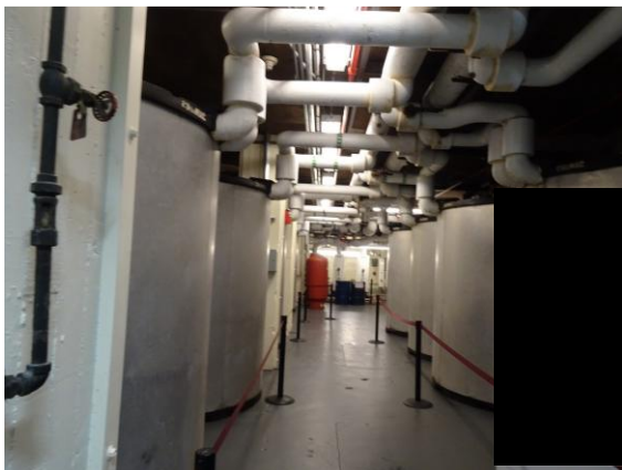
Ice storage system.
