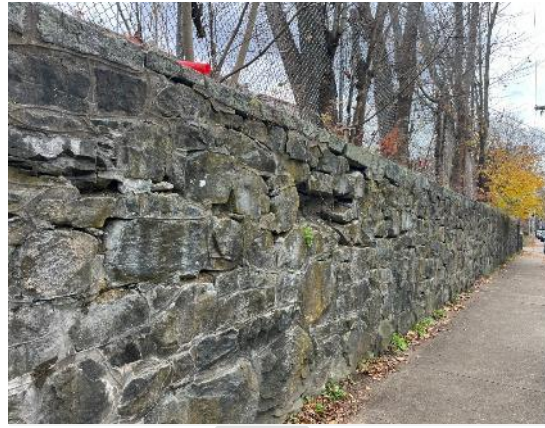
Degraded fieldstone wall along [REDACTED]
