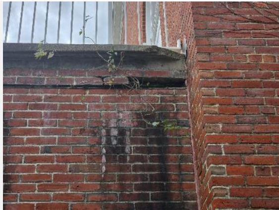
Displaced and damaged brick masonry where ivy was removed.
