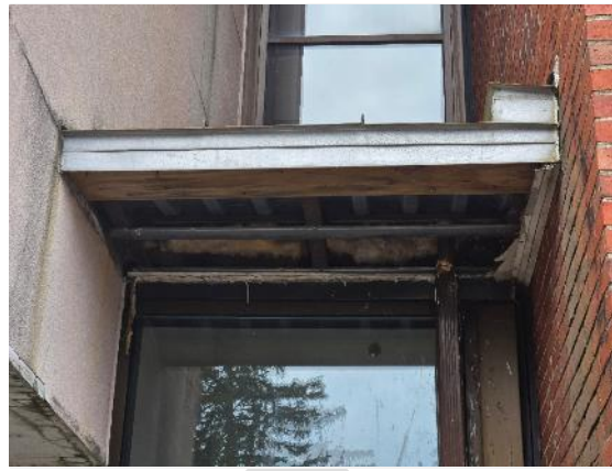
Damaged and missing soffit.
