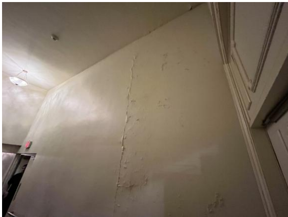
Typical water damaged observed along the North side of the building.
