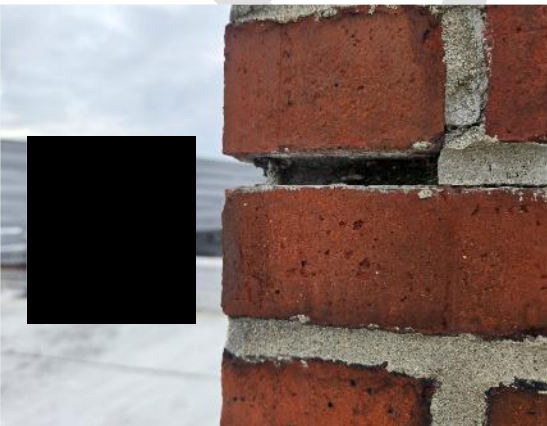
Failed pointing mortar.
