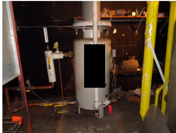
Domestic hot water boiler.
