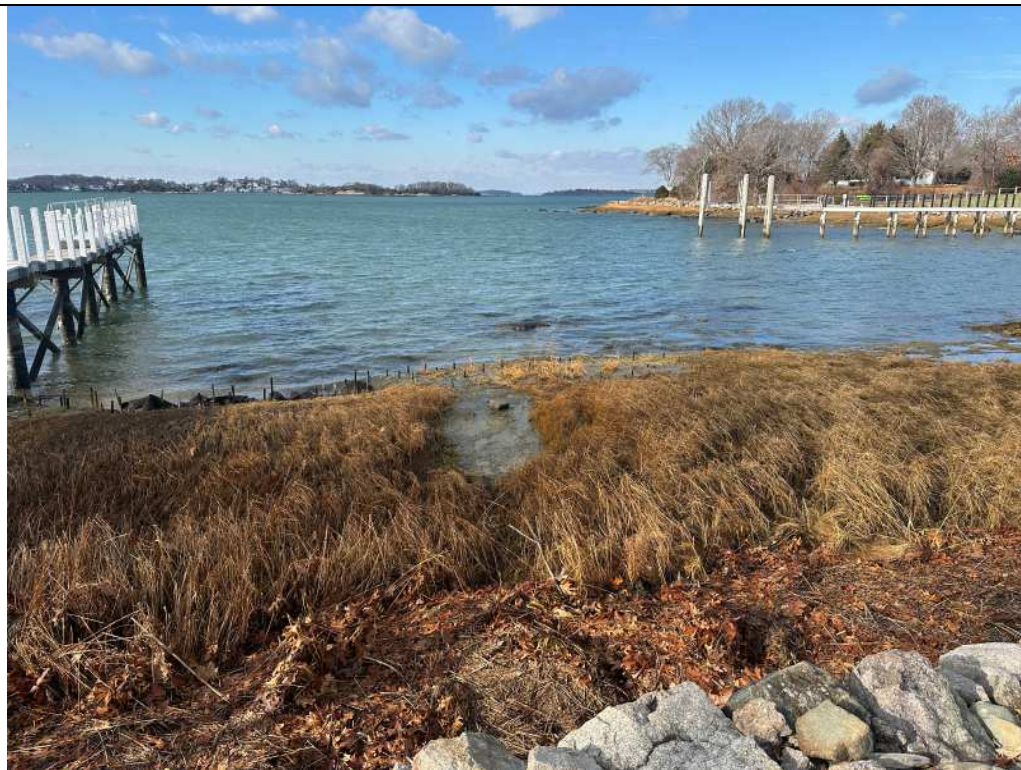
Northerly side of dock. 10'x3' area with no vegetation due to coir matting damage (requires replacement planting)
